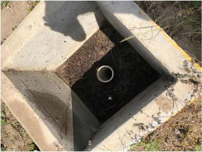
Figure 1. Monitoring well MW-1.
