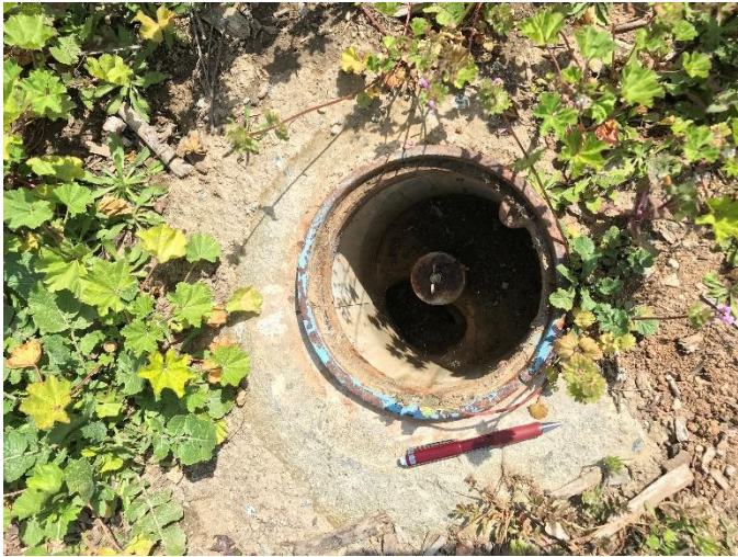
Figure 12. Monitoring well MW-5.
